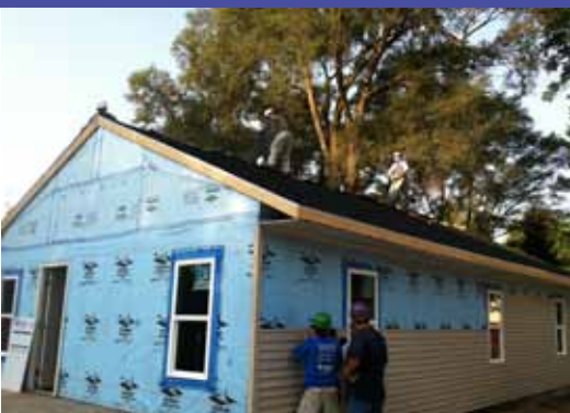
Installing blue board and partially recycled siding adds a layer of energy protection.
