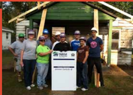
Volunteers caulk every air leak to make sure the home is energy efficient.
